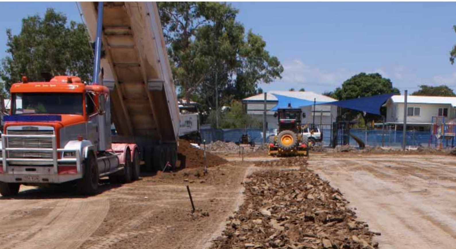
A quick glance shows this project is unravelling: delivering sub grade while ripping isn't an ideal scenario.
