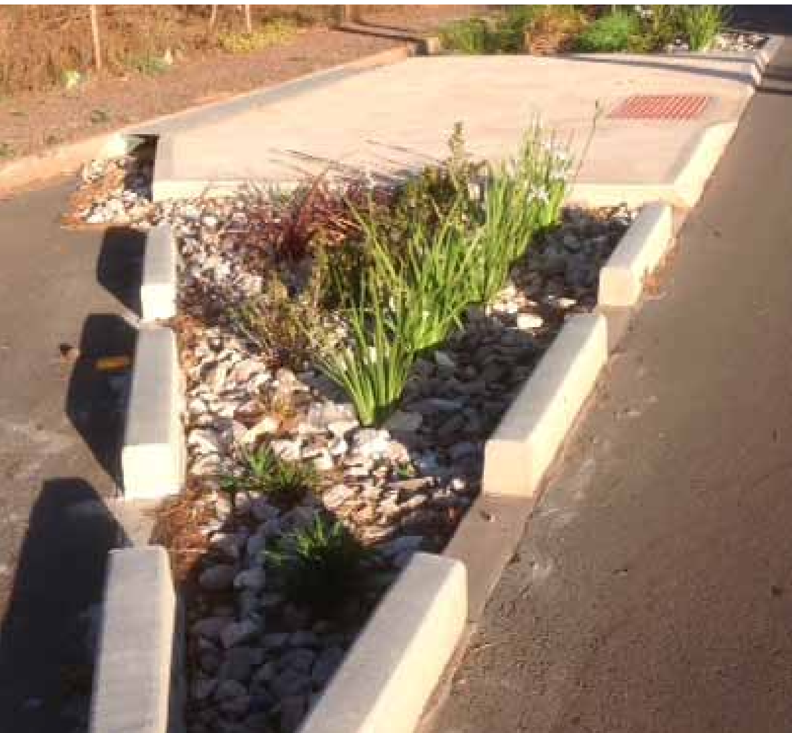
Check out the unique formwork which aims to take in as much storm water runoff as possible: the TerraCottem in the soil mix stretches it as far as possible between showers.
